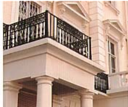
Inappropriate replacement of 'bottle' balusters with railings and crude simplification of stucco detail.
