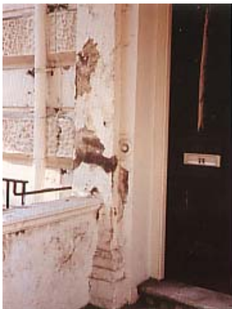
Example of badly deteriorating mid 19 th C stucco in the Westbourne area (photo 1988)
