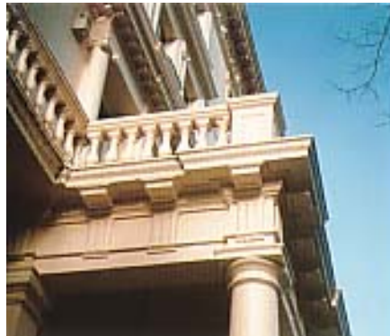
Recently restored balustrade and classical details to porch of stucco property in Bayswater.
