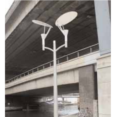
Lighting units on the canalside
